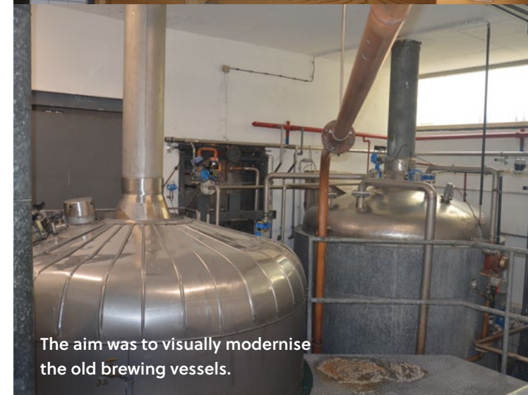
Now, a modern Braumat process control system replaces the former classic control panel.
